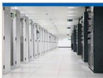
机电设备 ELECTRICAL EQUIPMENT
