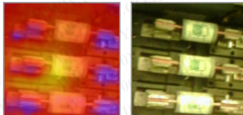
Detect issues with switchgears
